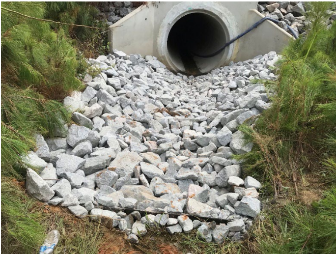
Lower Reach Additional Remediation – Sill and placed riprap at the pipe inlet (July 31, 2025)
